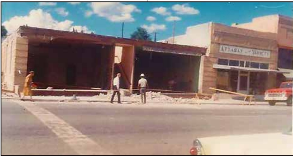
1966 construction on the First State Bank. The top story was removed from the vintage brick structure, everything modernized, and building extended to take in the Ataway building at right. First State became United Business Bank in 2019. The Hotchkiss Crawford Historical Museum has an extensive collection of historical photos.
