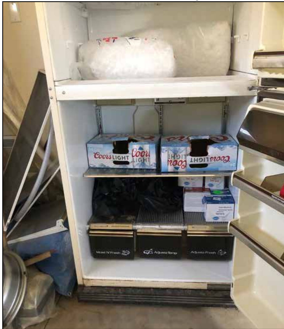
Water Plant Supplies Include Beer? According to former trustee Suzanne Watson a visit to a Town water treatment plant by one of the current trustees and others last September found the plant unlocked and an otherwise unsecured with no cautionary signage. A refrigerator there was observed to contain liquid alcoholic refreshments. (Photo shared by Watson taken by the trustee.)
