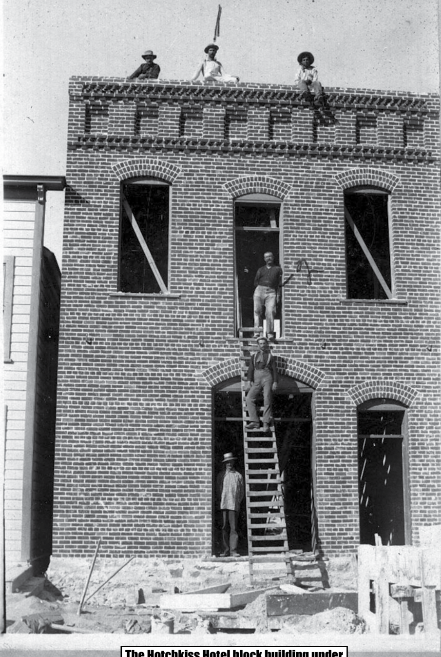
The Hotchkiss Hotel block building under construction in 1898 by the Sherman Brothers and Dwight Bennett and company Hotchkiss Crawford Museum collection photo
